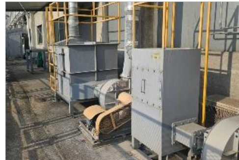
Air Pollution Prevention System
